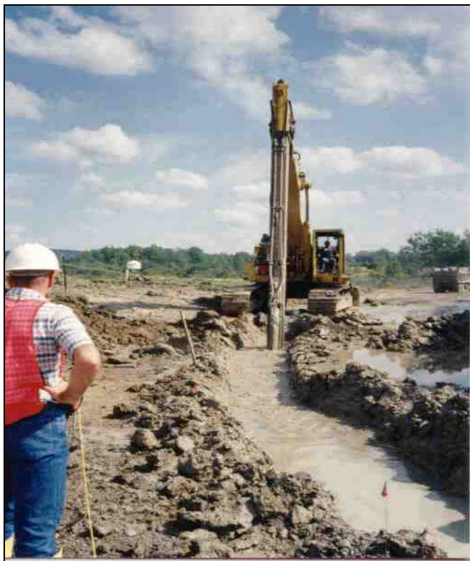
Construction of an underground slurry wall at a western New York landfill to prevent surface and groundwater contamination.
