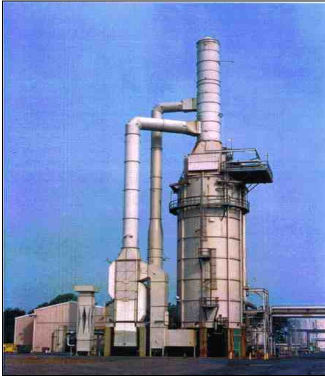
Hot oil furnace burning hazardous waste for energy recovery.
