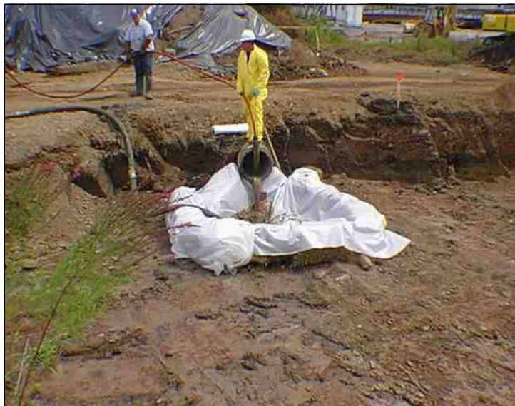
Restoration of wetland near Onondaga Lake by excavation of 12,000 cubic yards of PCB contaminated soil and flushing of contaminated sediment from sewer pipelines.
