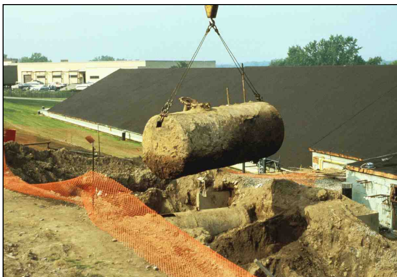
Deteriorating underground tank is lifted by crane in tank removal effort to prevent release into the environment.
