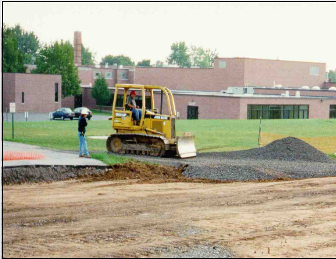
Excavation of 35,000 cubic yards of arsenic contaminated soils from a Niagara County school athletic field.
