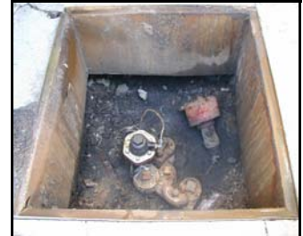
Uncontained turbine sump
