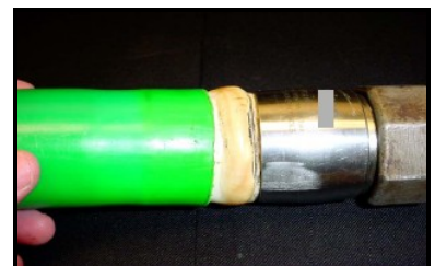
Flexible piping is bulging
