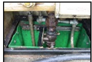
Contained dispenser sump
