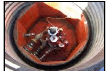
Contained turbine sump
