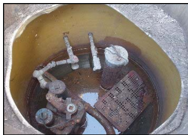
Contained sump with liquid and debris
