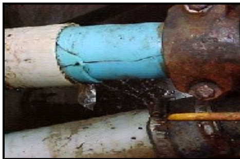
Flexible piping is cracked
