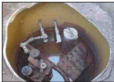
Contained sump with liquid and debris
