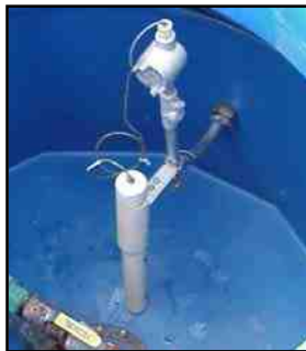
Float sump sensor
