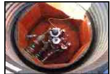
Contained turbine sump
