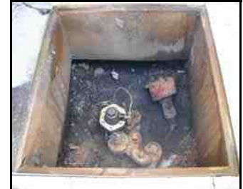
Uncontained turbine sump
