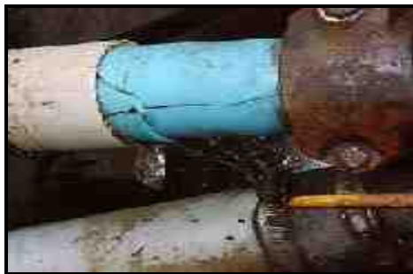
Flexible piping is cracked
