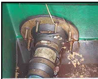
Sump penetration seals in poor condition
