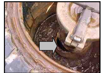
Spill bucket in poor condition – note the gap between the spill bucket and the fill pipe
