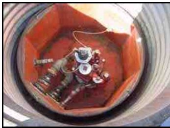
Dry, debris-free contained turbine sump
