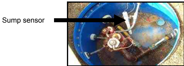
Sump sensor in contained turbine sump
