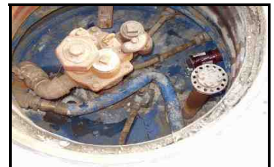
Flexible piping is kinked
