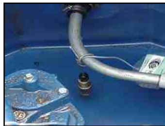
Liquid sump sensor
