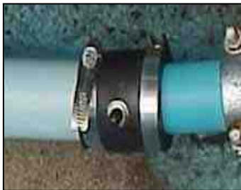
Test boot located in a sump
