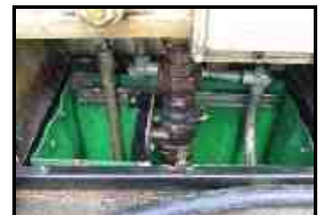
Contained dispenser sump
