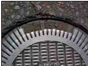
Cracked spill bucket lid
