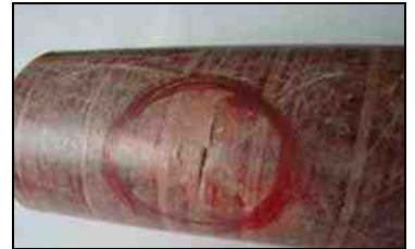
Fiberglass piping is cracked
