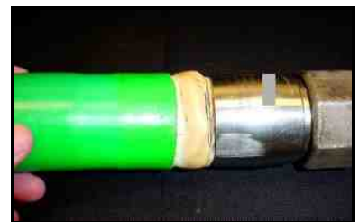
Flexible piping is bulging
