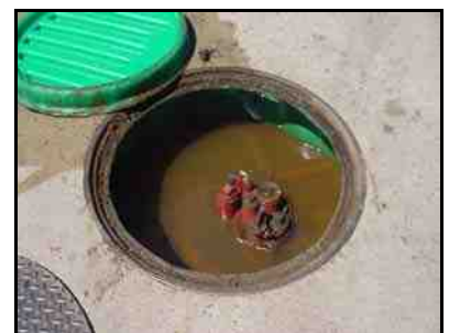
Contained turbine sump full of liquid
