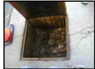
Square steel sump lid pulled up to show the inside of an uncontained turbine sump
